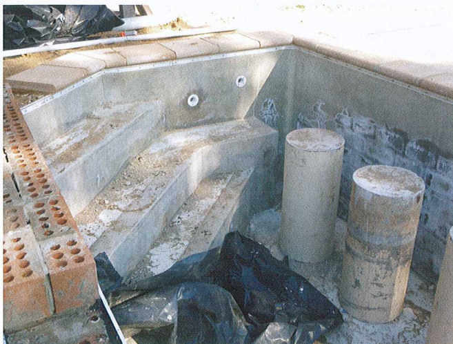
The concrete shell of the complex pool that is yet to be adorned with an Abgal custom-made liner
